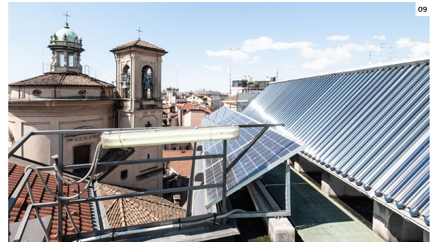
– 09 Milan, Italy Solar panels installed on roof
